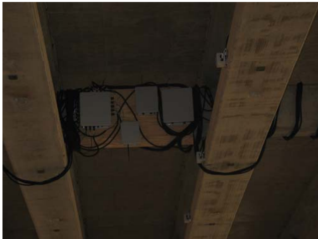
Fig. 7: The Bridge Monitoring System at Canadian River Bridge
